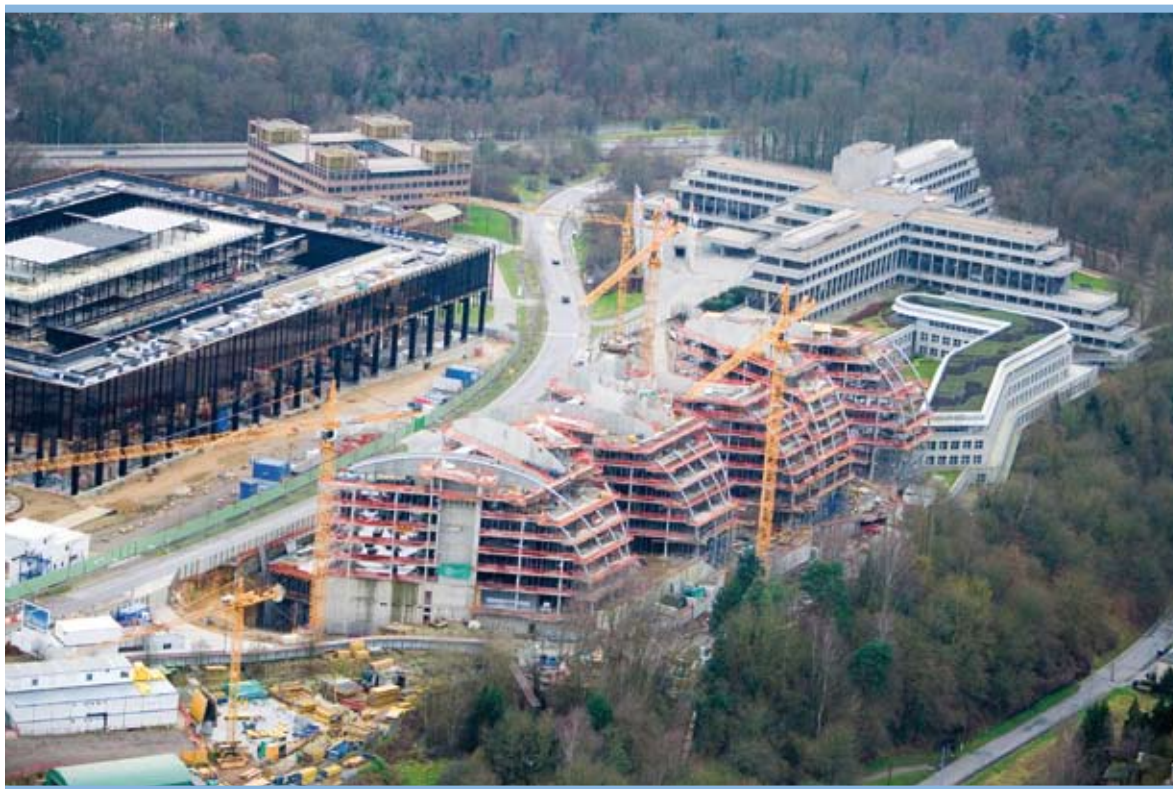
This view from the north shows work in progress on the EIB's new building (foreground) in September 2006.
